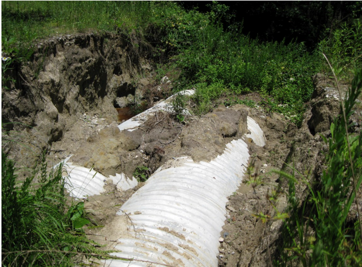
Figure 13. Exposed culvert pipes in the Athol Complex after extreme flooding washed out the road in 2013.
