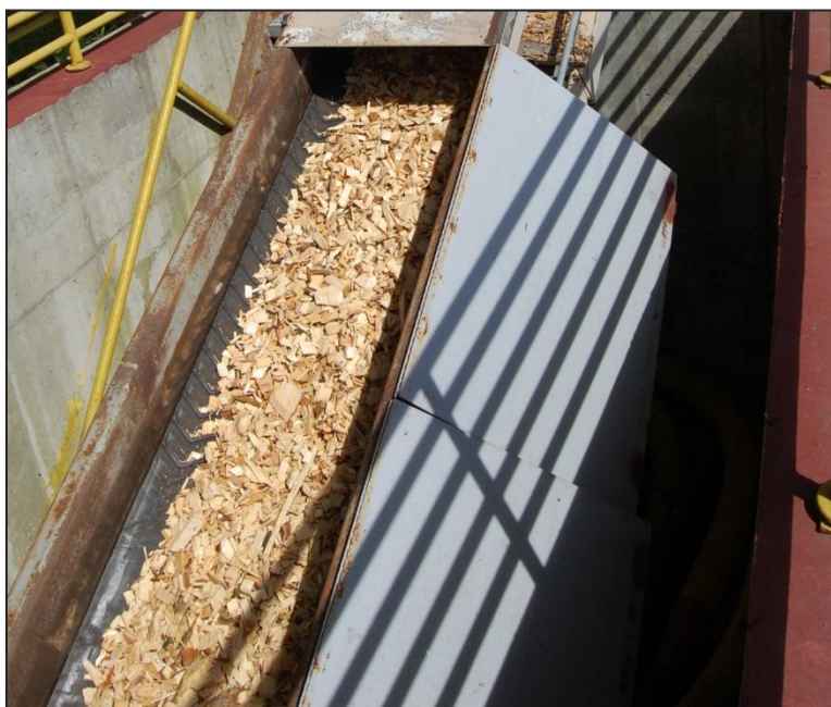
Woodchip conveyor at a biomass-fired CHP facility.
