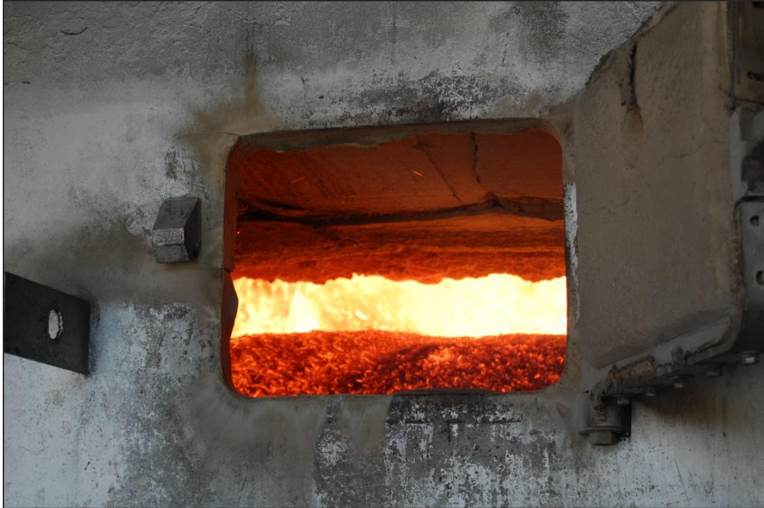
Biomass combustion in a 2 MW boiler.
